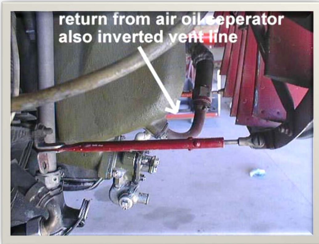
Figure 5. Separator Return Line (Oil Return Nose Case Fitting P/N 526200-50W)
